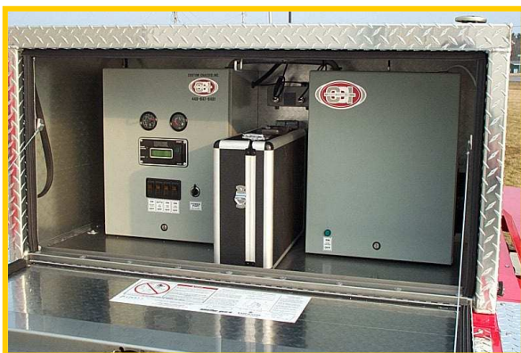
Curbside mounted control panel with locked door.
