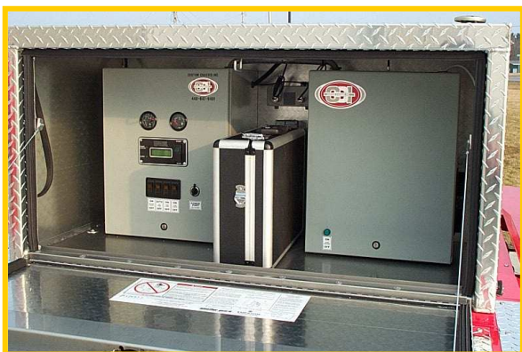
Curbside mounted control panel with locked door.
